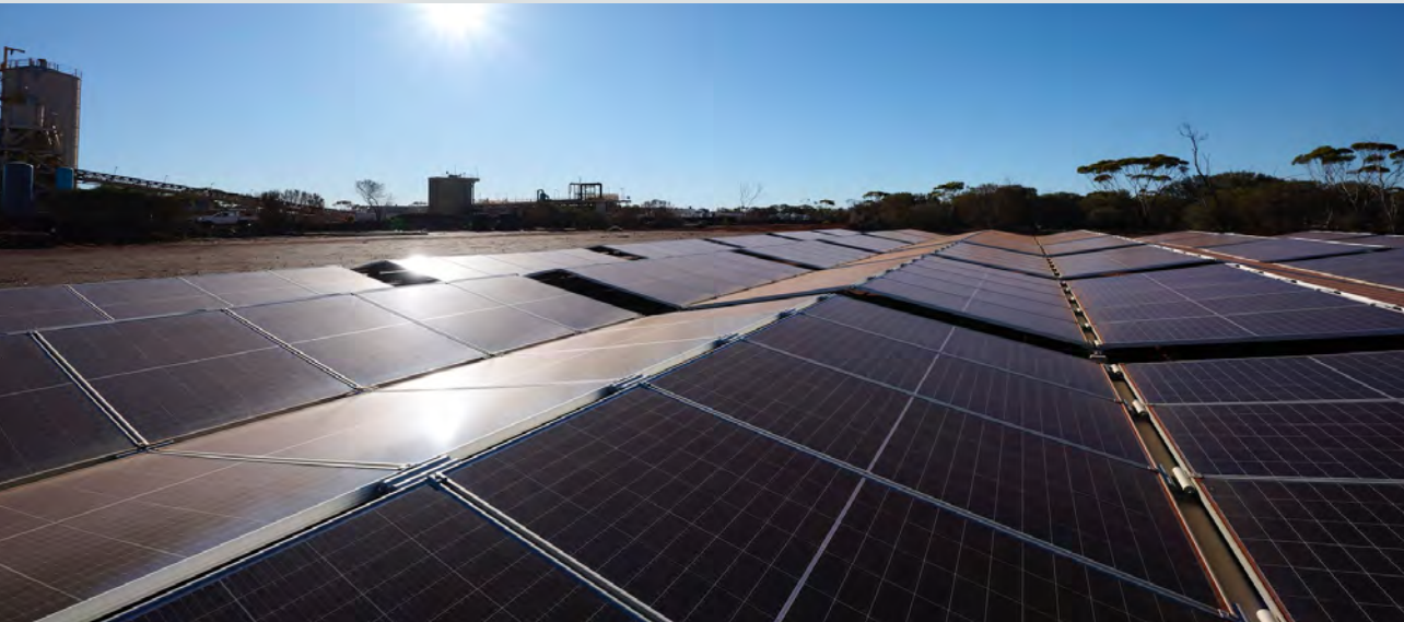
Figure 6 Existing solar array at Carosue Dam Operations
